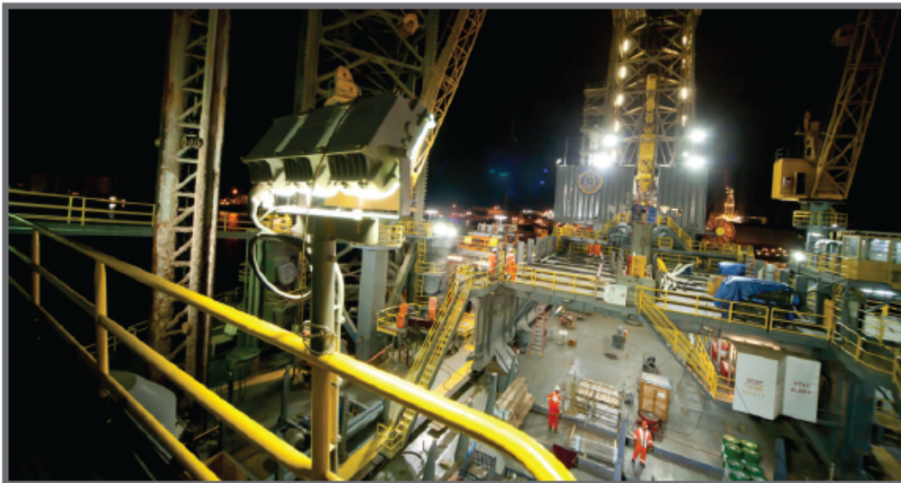
Oil & gas terminal lighting
